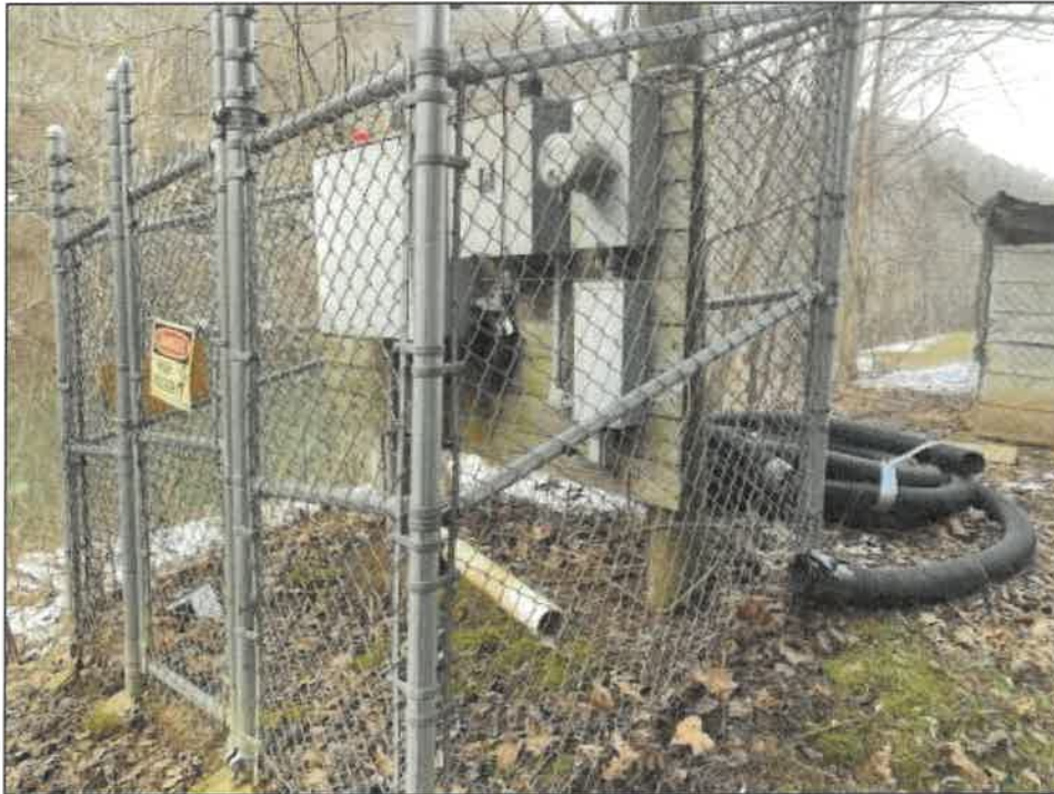
Pump Station No. 4 – also known as "Junior Gray Station" (Lat 38 27'23", Long -81 5'24")
