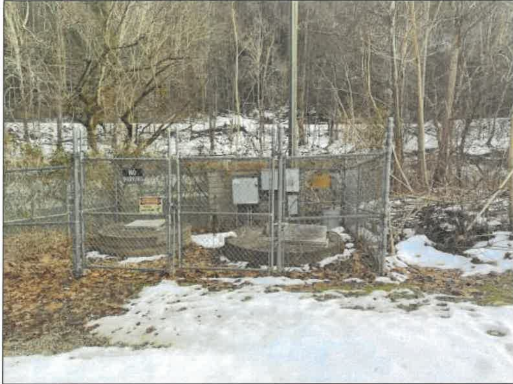
Pump Station No. 7 – also known as "High School Station" (Lat: 38 26'43", Long: -81 5'36")
