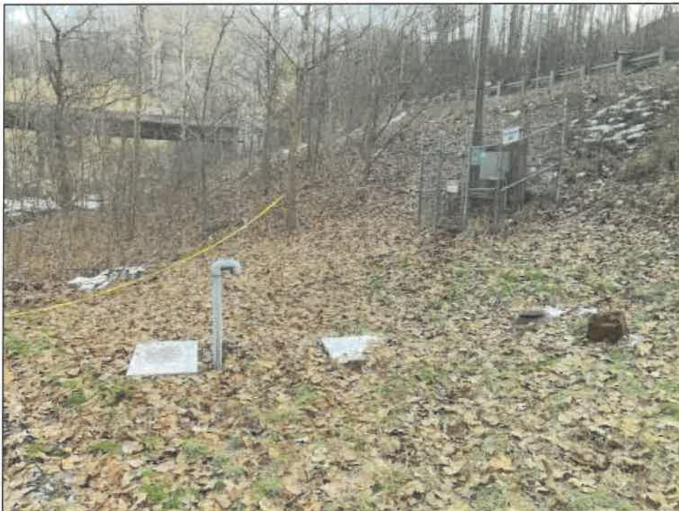
Pump Station No. 2 – also known as "Water Treatment Plant (WTP) Station" (Lat: 38 27'50", Long: -81 4'29")
