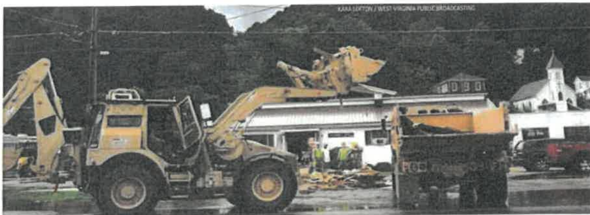
Image 23: Cleaning up flood damage in Richwood.
