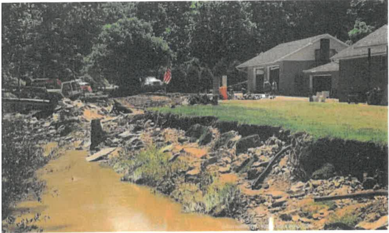
Image 25: An excavator, left, attempts to rebuild the piece of land where a private bridge used to sit. The bridge was washed away by flood waters.
