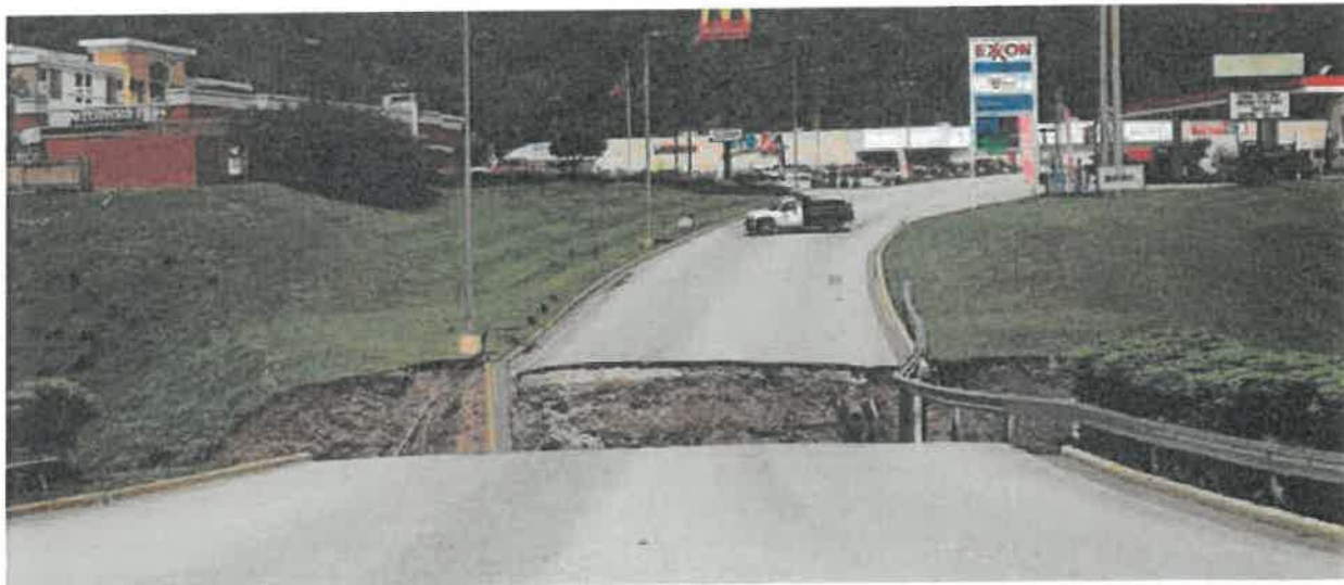
Image 20: Collapsed bridge at the Crossings Mall in Elkview
