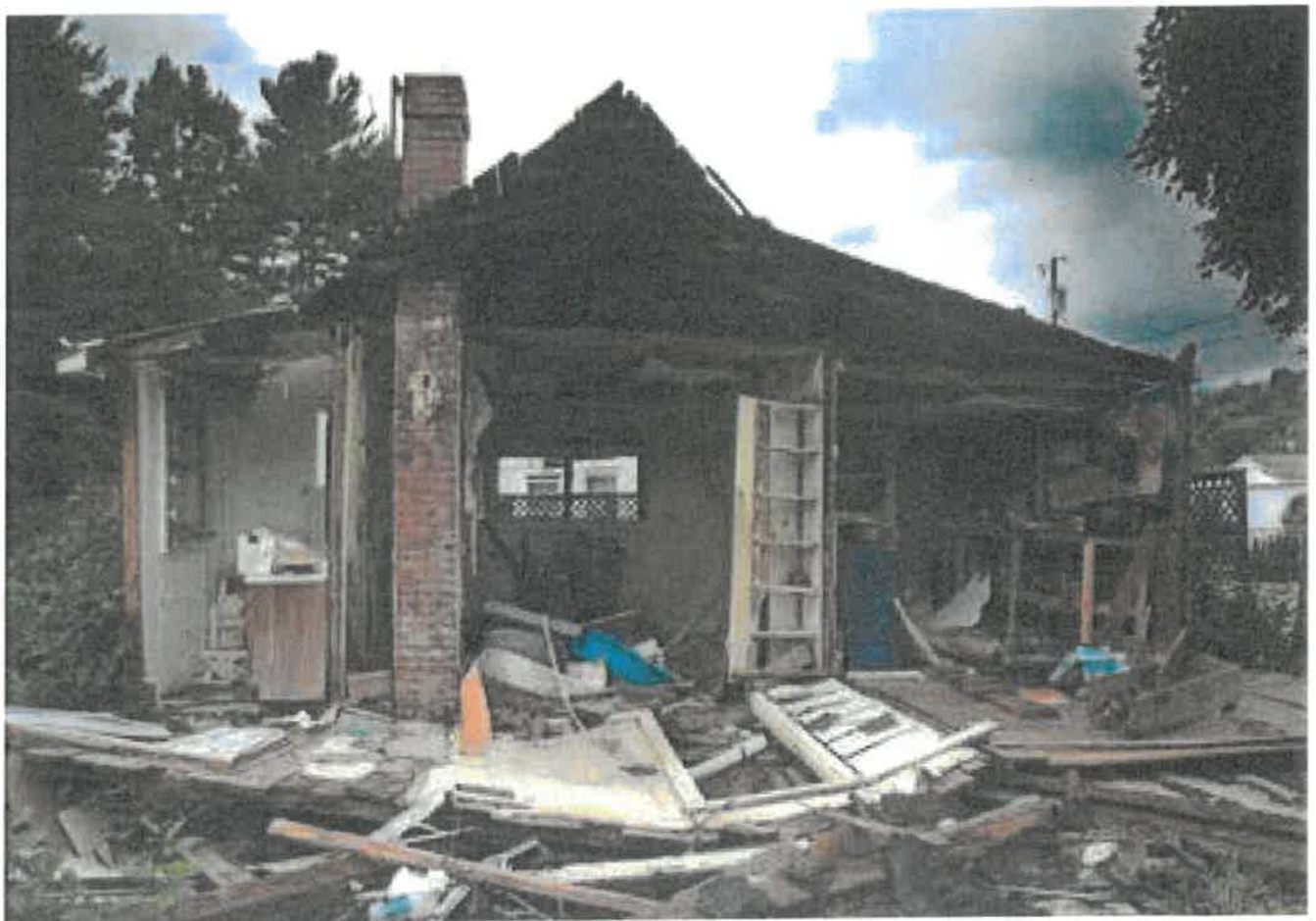
Image 10: A home destroyed by flood damage.
