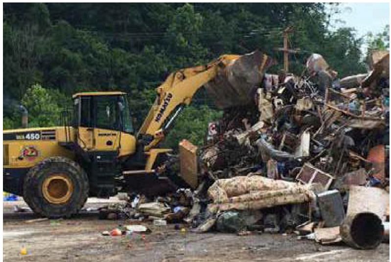
Image 19: Flood debris being removed off I-79's Clendenin Exit
