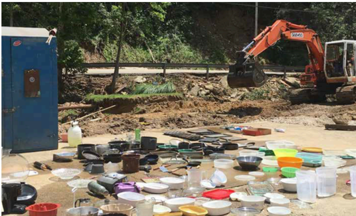
Image 1: An excavator rebuilds where a private bridge once stood while containers from a flooded kitchen are laid out to dry
