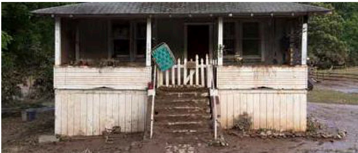
Image 18: Damaged home in Clendenin
