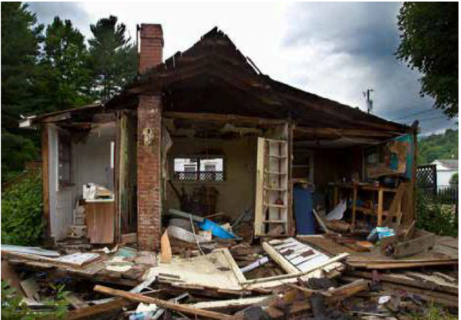
Image 10: A home destroyed by flood damage.
